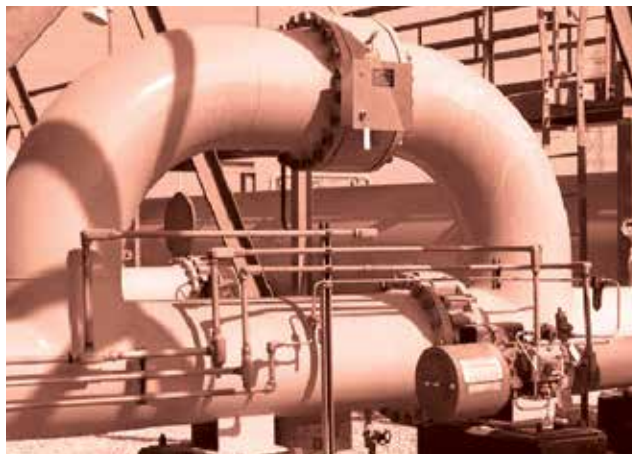
API 537 Compliant Application
